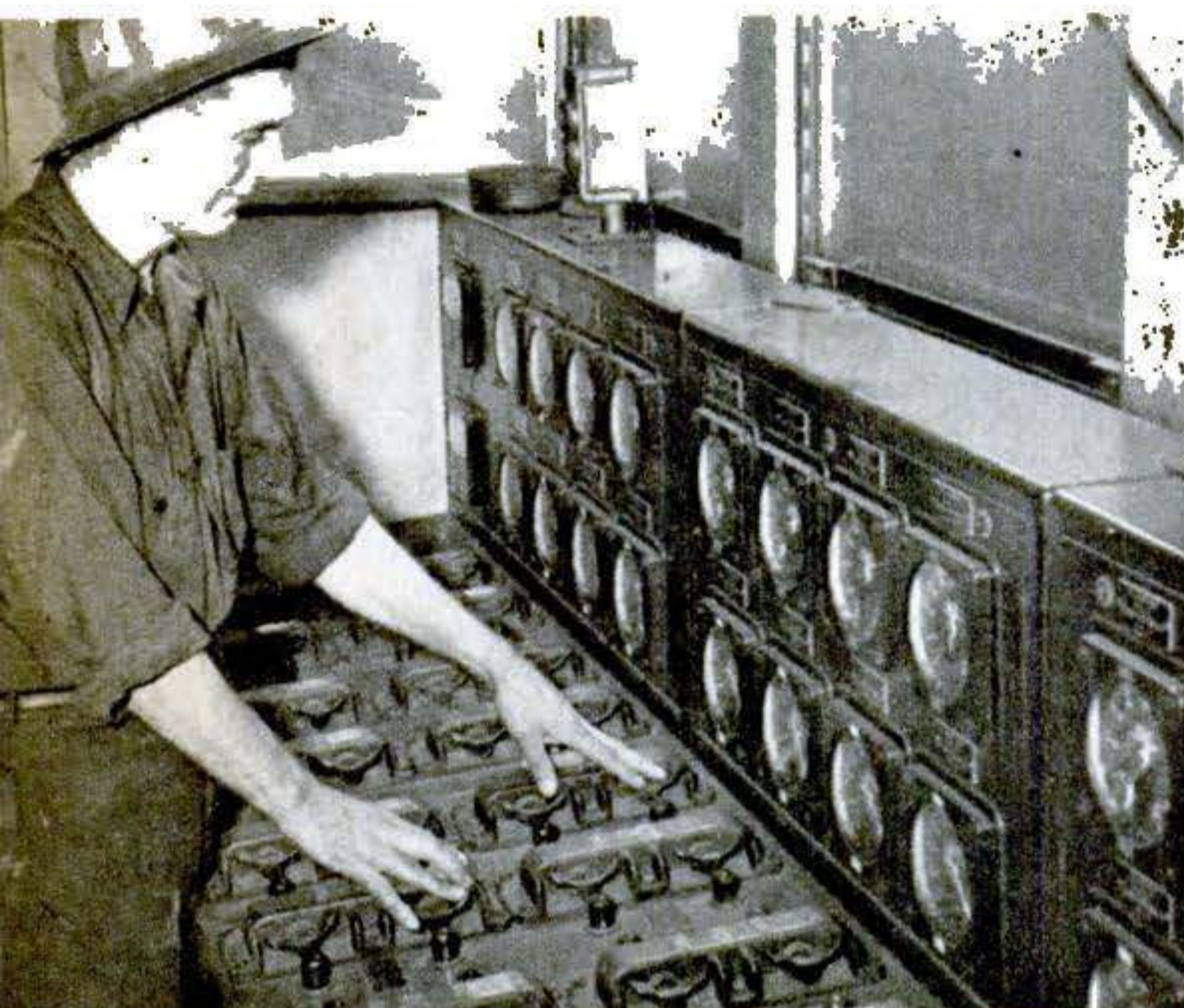
5. In control room on dock, operator flicks electric switches actuating pumps, valves. Pumps empty buoyancy compartments and dock rises at rate of one foot in 45 seconds, lifting the big ship bodily. Water around vessel spills from open ends of rising dock.
